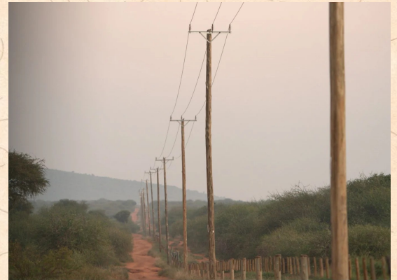
Laikipia powerline, ©Darcy Ogada
